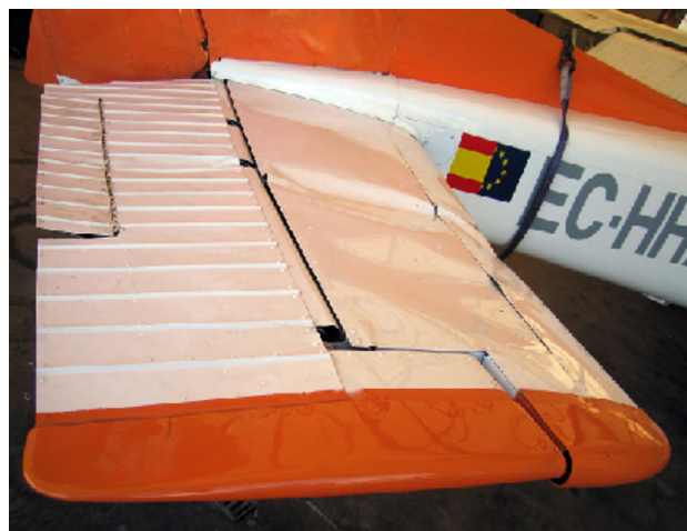
Figure 1. Damage to right stabilizer
