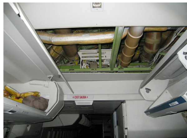
Figure 4. Main cabin overhead
